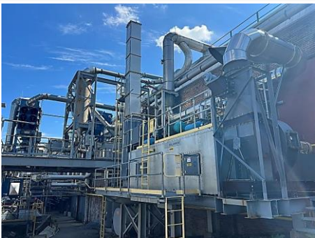
View of Dust Collectors in Courtyard
