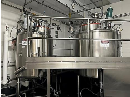
(2) Mueller 250 & 500 Gallon Stainless Steel Jacketed Mixing Tanks
