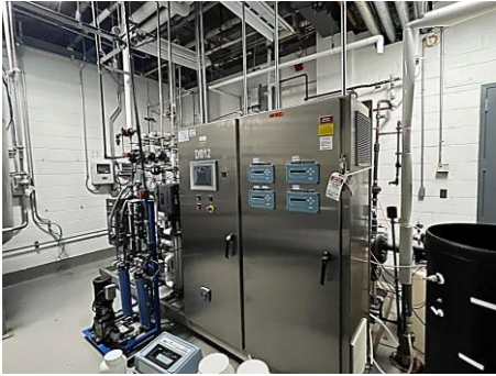
US Filter DI Water System Skid
