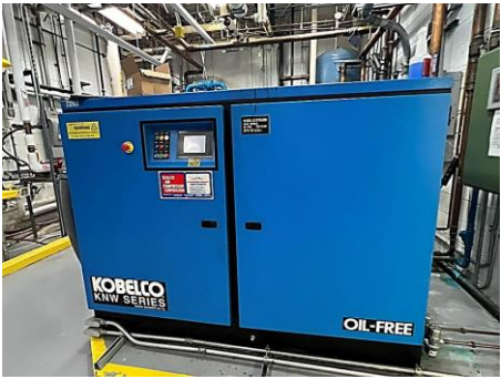
(2) Kobelco 200HP & 60HP Air Compressors
